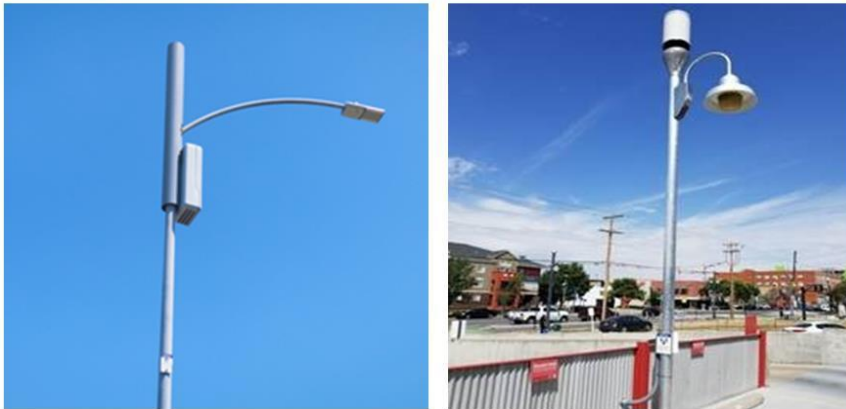
Figure 2. 5G equipment: Due to its small size, it has been installed on standard metal poles [11]
